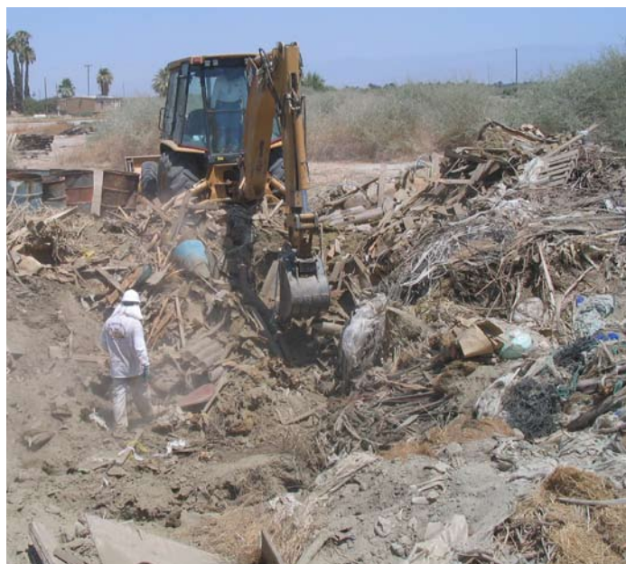
Buried debris and drums found in illegal pit behind a foreclosed manufacturing facility. Fortunately for the bank, hazardous materials were not present.
