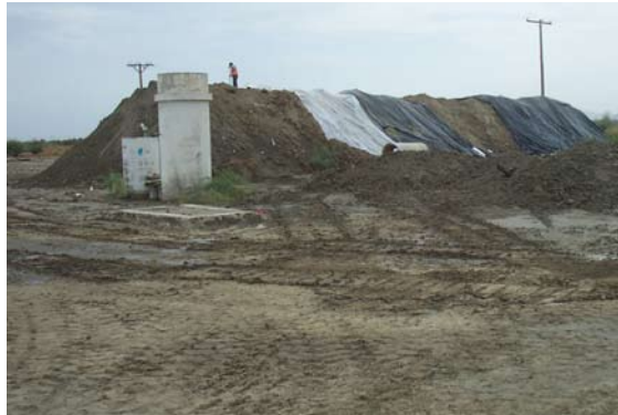
A stockpile of DDT-contaminated soil created by removing the top six inches from a two-acre area. Disposal cost: $600,000.
