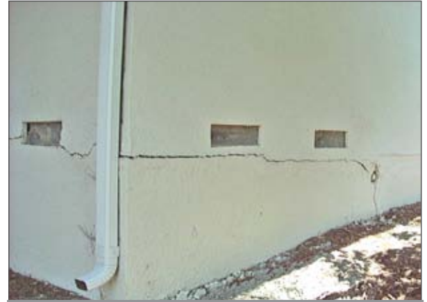
Foundation damage due to soil expansion
