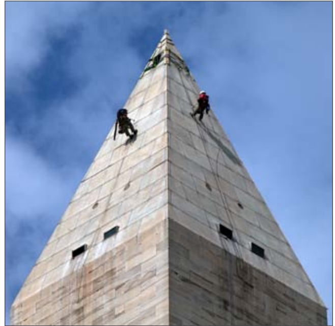
Contractors from WJE conducting exterior assessment of the Washington Monument on September 28, 2011. Over 555 feet tall, the free-standing masonry structure sustained damage such as cracks and displaced stone.
