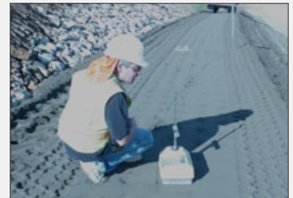
Alex tests the density of soil cement at the Santa Maria Levee Improvement project
