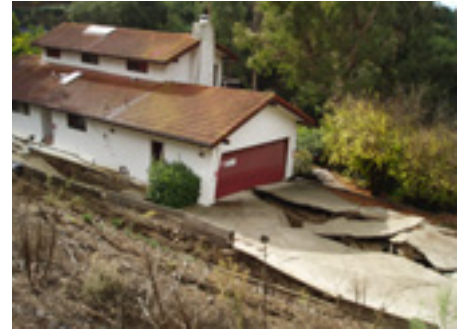
Sycamore Canyon home damage.
